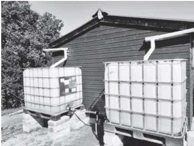
Our current IBC system holds 2000 litres of water collected from the shed roof
